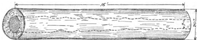
FIG. 4.—Deduction for defect caused by center or circular rot
